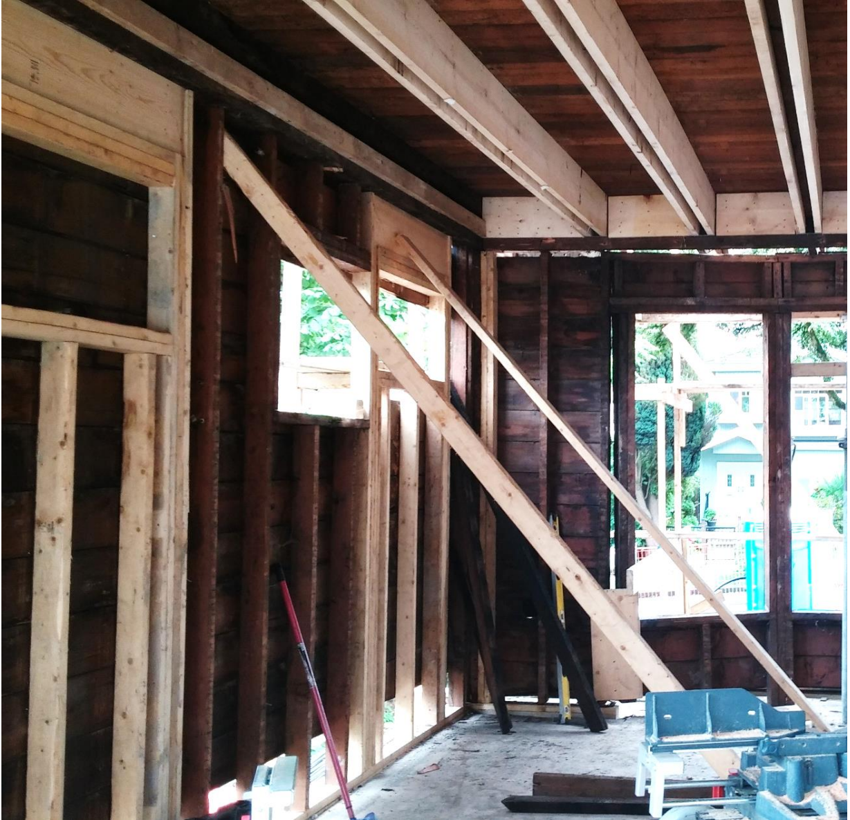
Figure 41 Old studs and joists of a heritage house supported by new lumber for structural purposes
