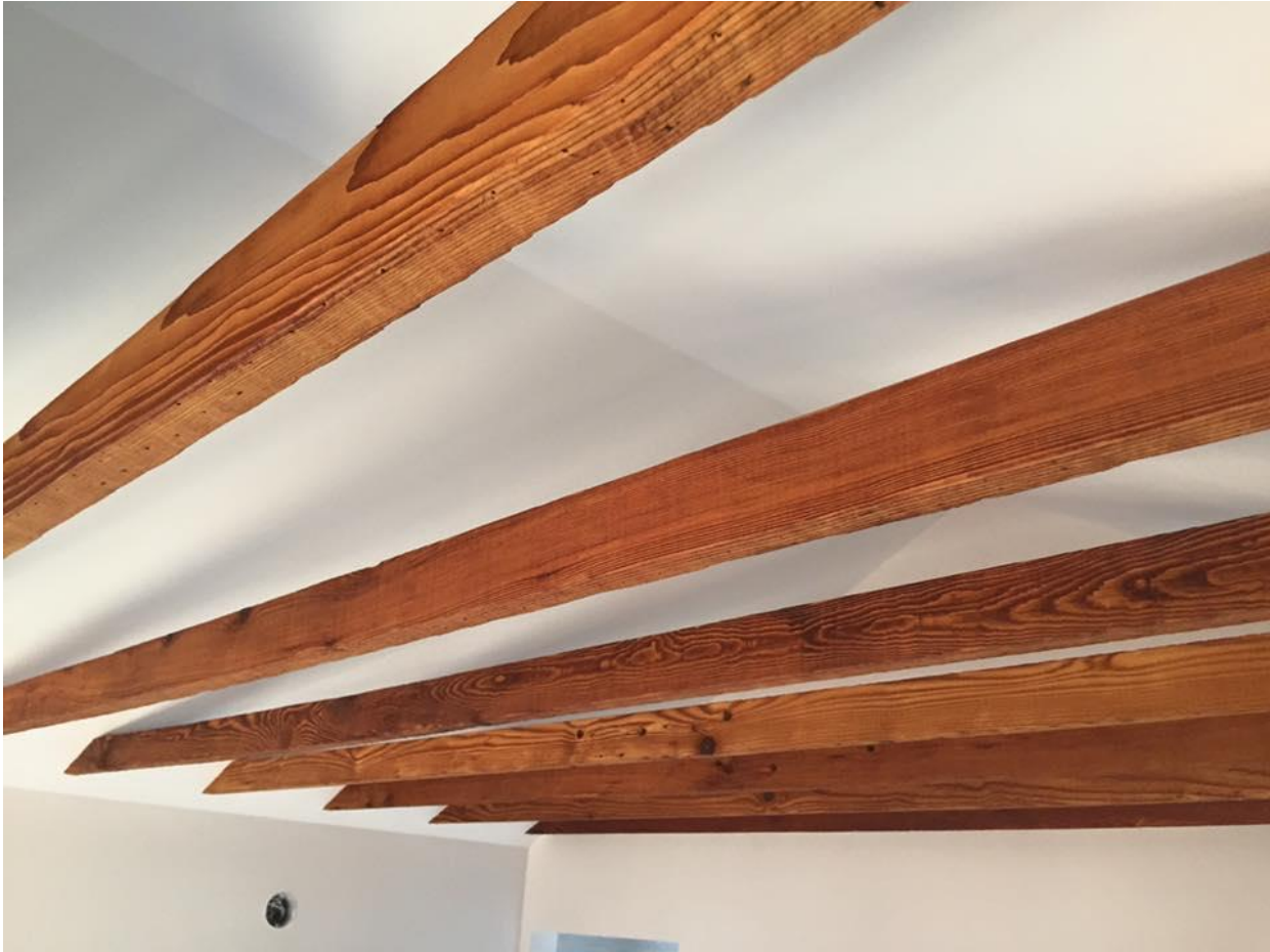
Figure 40 Ceiling joists kept exposed in renovation for aesthetic purposes ( Naturally Crafted Construction )
