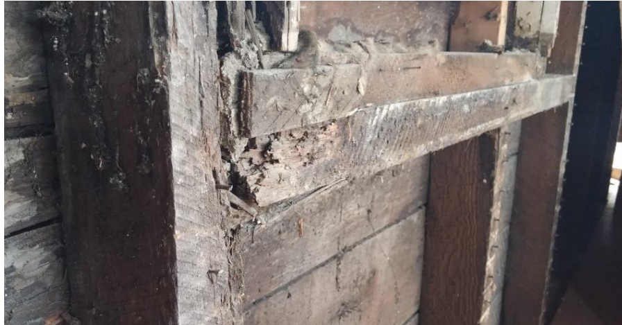
Figure 5 damages in lumber used in a 1920s house
