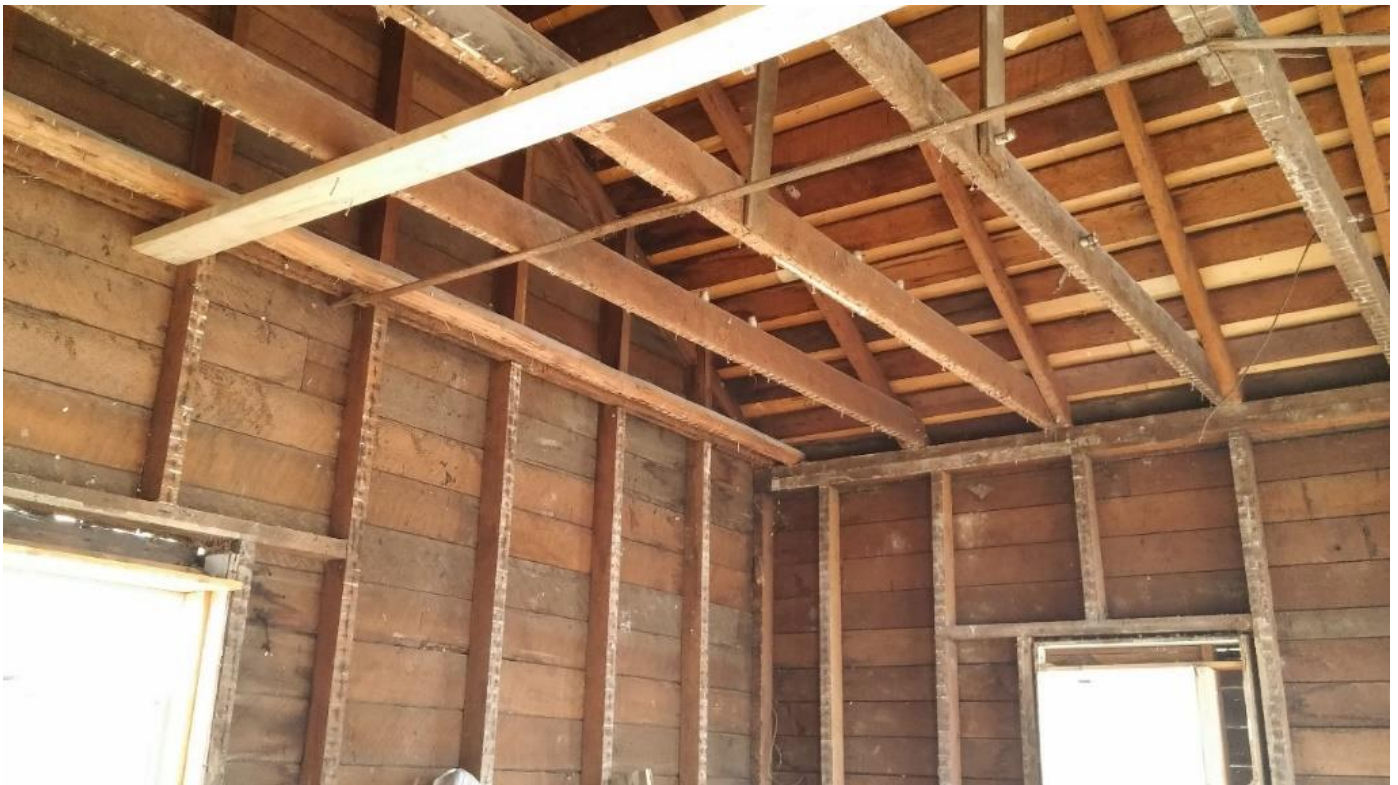
Figure 4 Framing structure (2×6 joists and rafters, 2×4 studs, and sheathing) of a 1920s house
