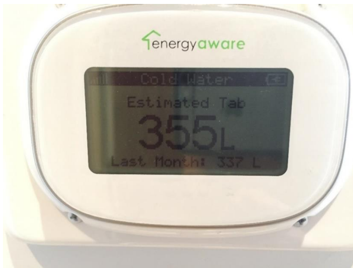
Figure 17. An in-suite monitor that shows the monthly cold water consumption of a unit at Olympic Village (photo courtesy: Andrew Ling).
