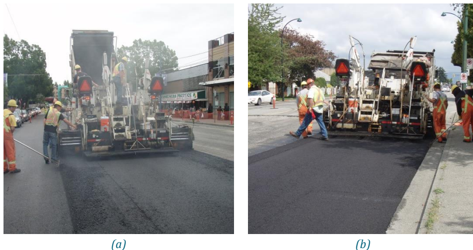
Figure 8: HMA versus WMA visual comparison; (a) HMA, (b) WMA (Photos courtesy of Kent Yard)
