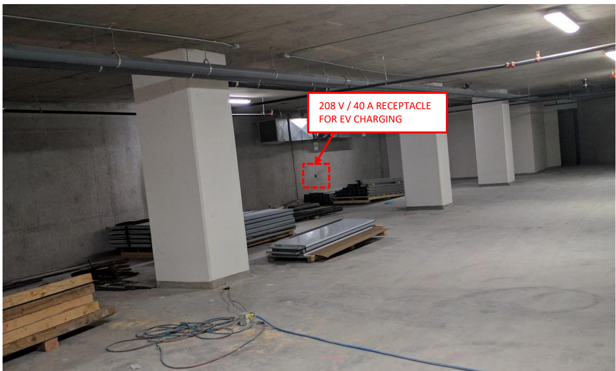
Photos 10 and 11: A view of two distinct levels of the multi-level underground parkade, wherein 20% of the parking stalls are provided with dedicated 208 V / 40-A EV charging outlet boxes.
