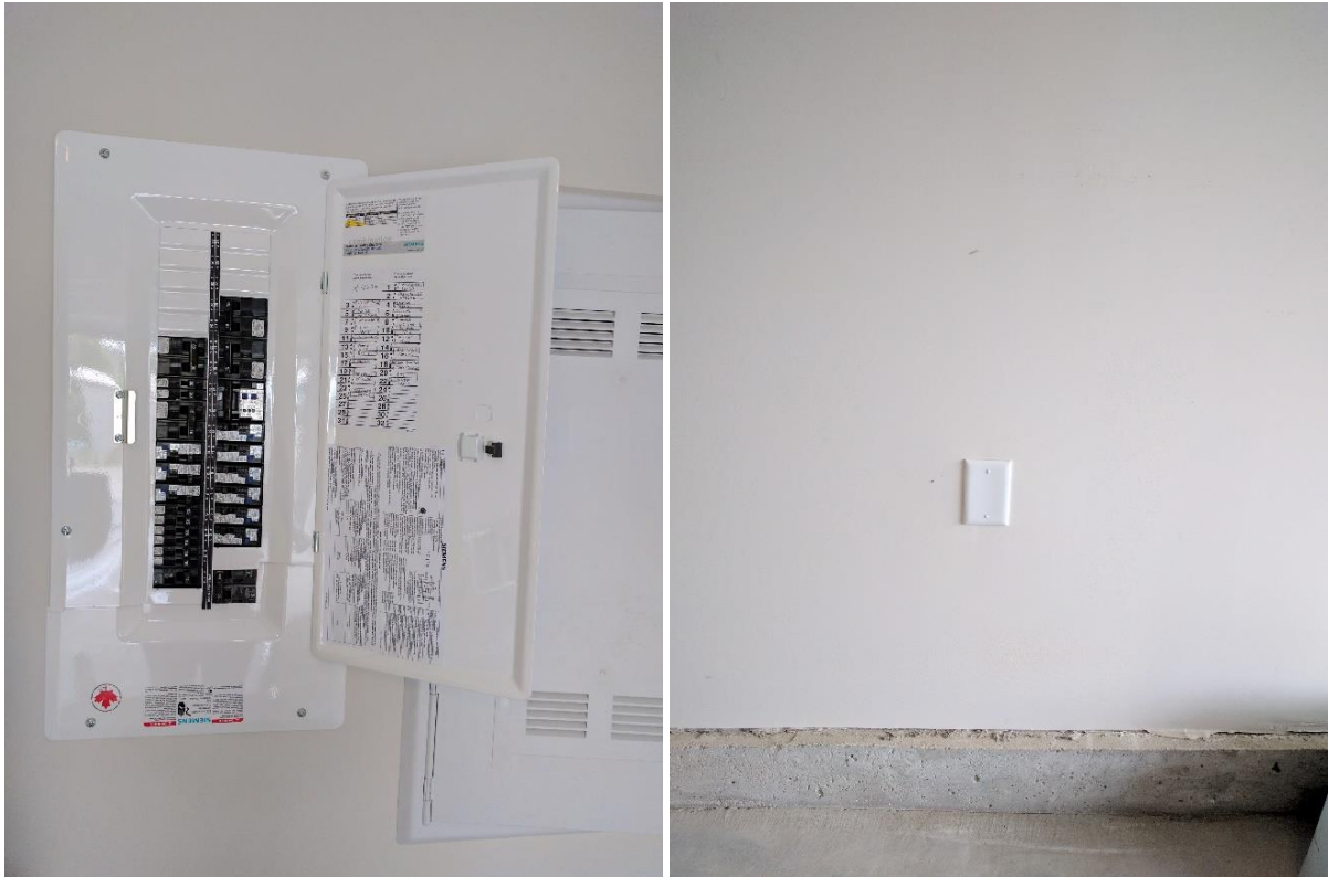
Photos 5 and 6 (L-R): An internal view of the local electrical panel, located at the parking stall, supplying a dedicated outgoing branch circuit capable of supplying 240-V / 40-A to the EV charging outlet box; A close-up view of the outlet box mounted on the wall.
