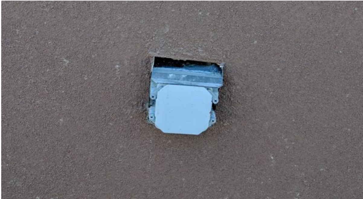
Photo 5: A view of the EV charging outlet located at the on-grade parking area.
