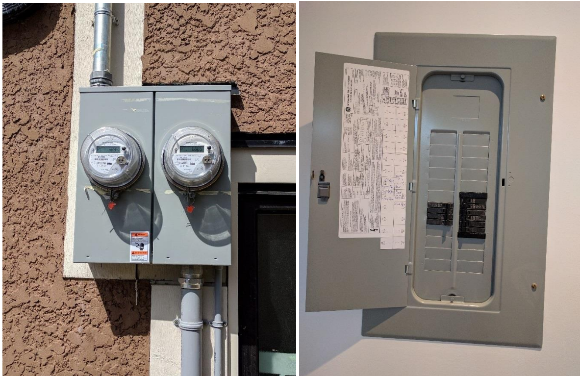
Photos 1 and 2 (L-R): An external view of the LV metering for the incoming electrical supply at the Laneway House; An internal view of the main electrical panel, fitted with a dedicated outgoing branch circuit capable of supplying 230-V / 40-A to an outlet box at the parking garage.
