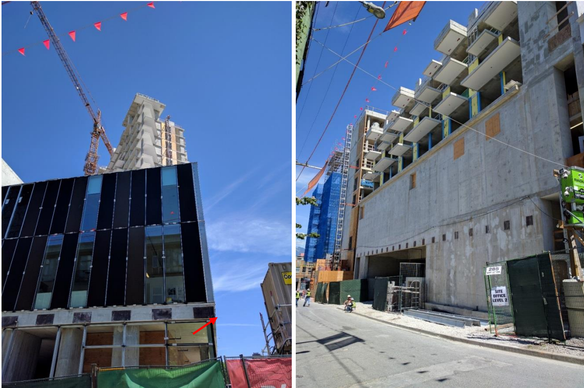
Photos 2 and 3: A view of the mixed-use building under construction at 285 East 10th Avenue.
