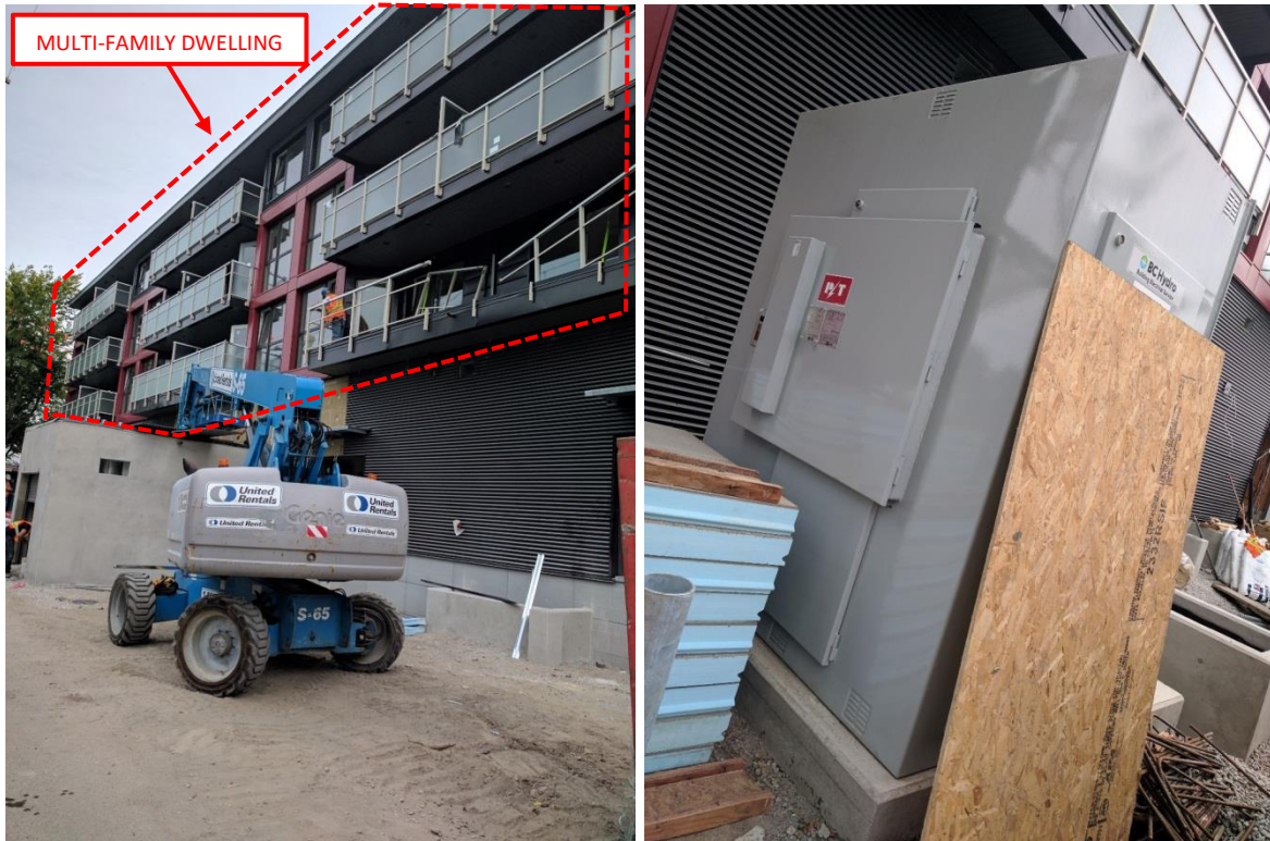
Photos 2 and 3 (L-R): A view of the mixed-use building located at 1720 Kingsway; An external view of the incoming 12.5-kV supply cubicle provided by the electric utility (BC Hydro).
