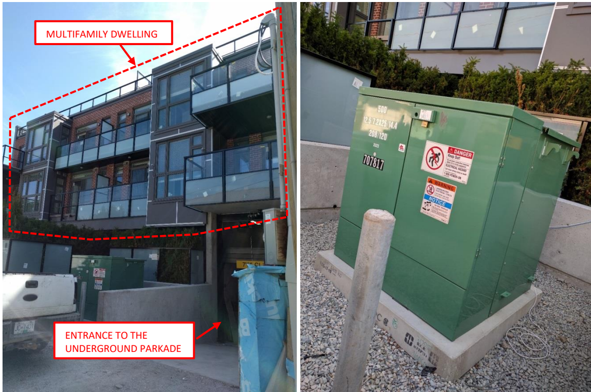
Photos 2 and 3 (L-R): A view of the mixed-use building located at 3939 Knight Street; An external view of the incoming 12.5-kV supply cubicle provided by the electric utility (BC Hydro).
