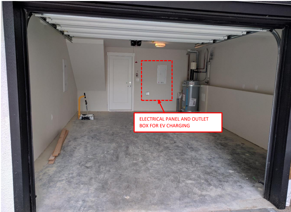
Photo 7: A view of one of the parking stalls fitted with EV charging infrastructure.
