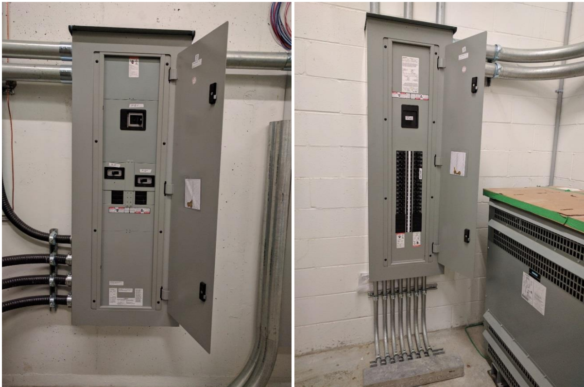
Photos 4 and 5 (L-R): A view of the main electrical panel, located within the electrical room, supplying “P1EV” - a dedicated panel supplying charging infrastructure for Electric Cars and Bikes; An external view of the panel “P1EV”, located within the electrical room, fitted with dedicated outgoing branch circuits capable of supplying 240-V / 40-A to the EV charging receptacles at the multi-level underground parkade.
