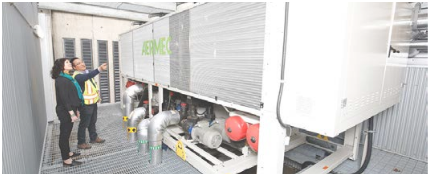
Vancouver City Hall heat pump, City of Vancouver
