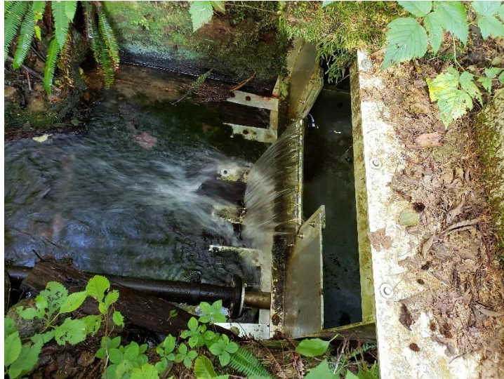
Figure 9 – Seymour Dam run-off 18" drain
