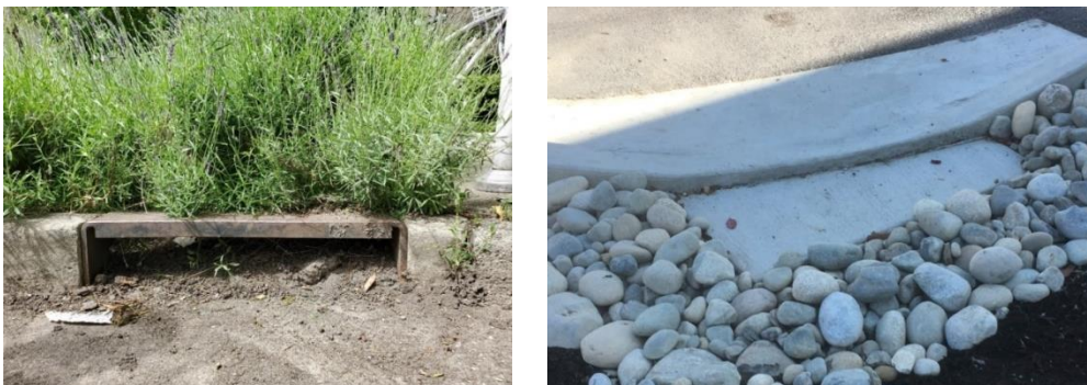
Figure 30: Street side bioretention inlet clogged without pretreatment and an inlet with sediment pad and drop behind the inlet that reduces potential for clogging and eases maintenance
