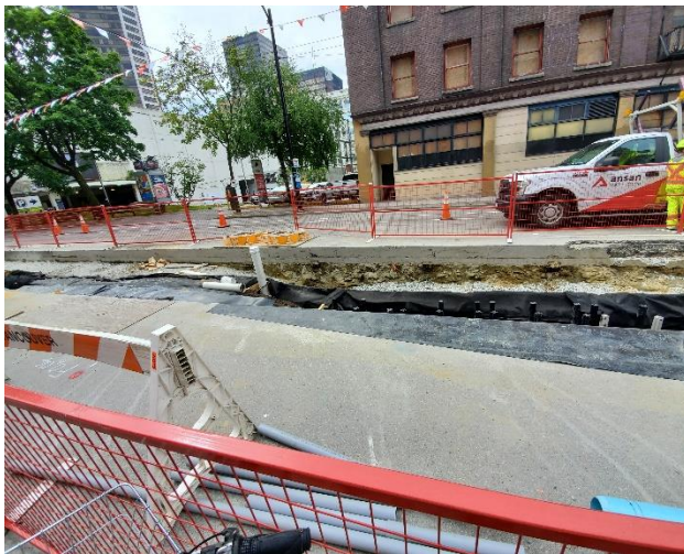
Figure 26: The construction of subsurface infiltration component underneath a bike path in Downtown Vancouver, Richards and Dunsmuir.
