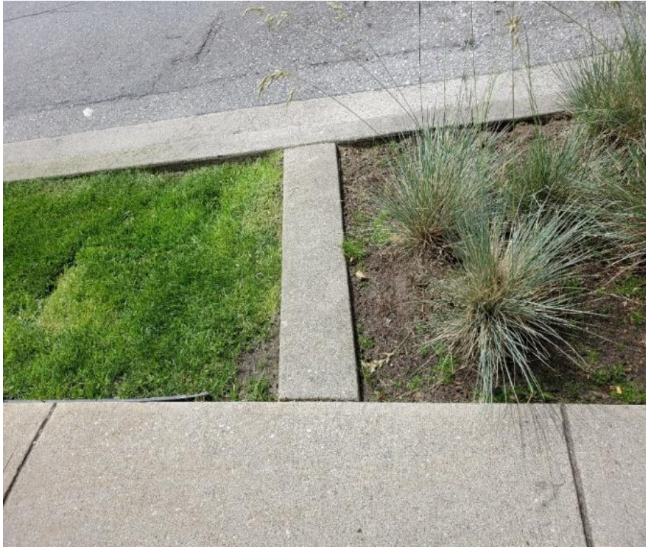
Figure 34: Barrier used to separating bioretention vegetation from grassed boulevard helps to prevent vegetation creep from one area to the other, Pine St, Vancouver, BC, June 2020.
