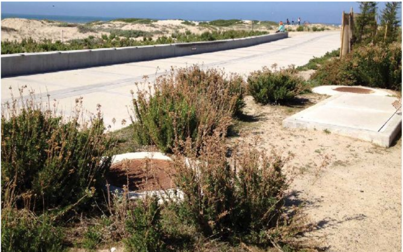
An 8' x 24' Stormwater Management StormFilter with 60 cartridges is used to remove pollutants from runoff at Surfers Point Beach in Ventura, California (Contech, 2020)
