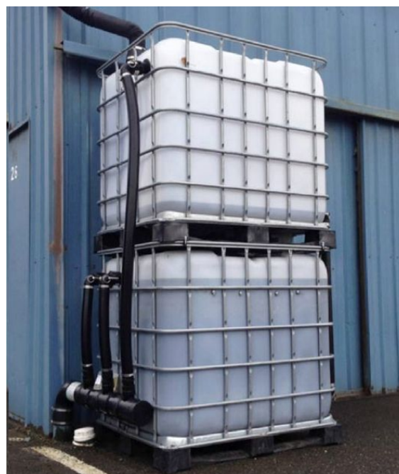
Pilot scale Downsprout filter at the PoPT facility (Gray et al., 2015)
