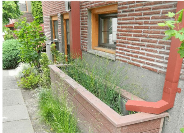
A disconnected downspout (Campos et al., 2015)
