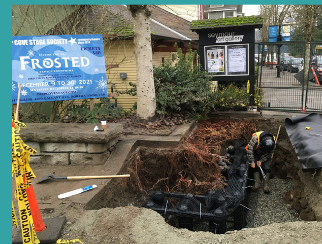
Figure 3.6: Installing Silva Cells and carefully folding the roots of the preserved Bowhall maple tree into the cells to provide access to increased soil volume. Source: from Deeproot (n.d.).
