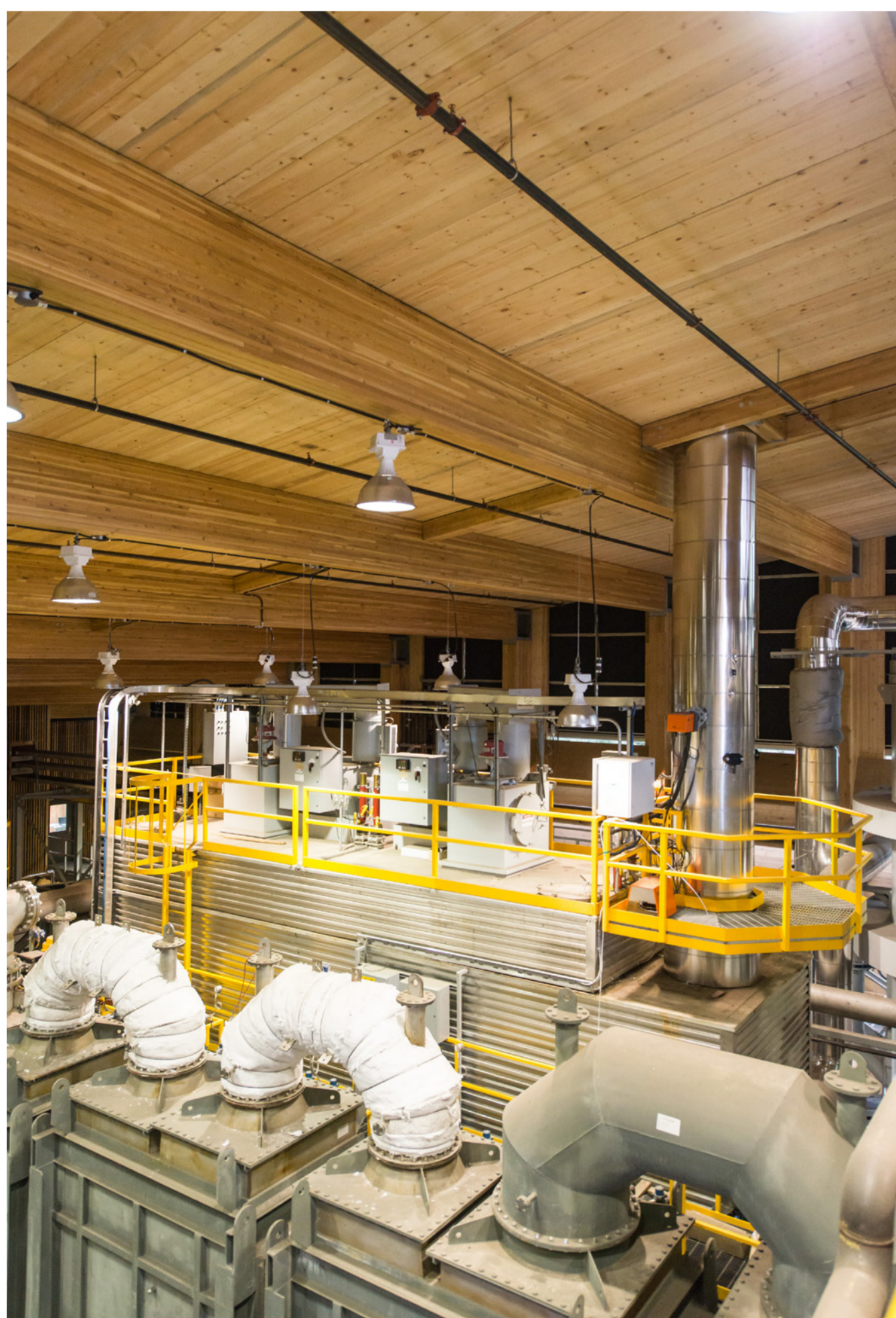
Thermal system within the BRDF
