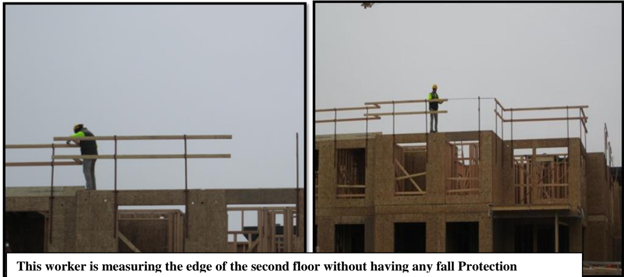
Figure 7: Safety Issue - Fall Hazard
