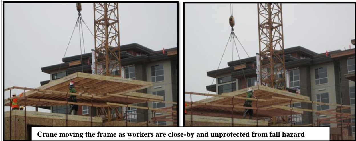
Figure 9: Safety issue – Crane Operation and Fall Hazard
