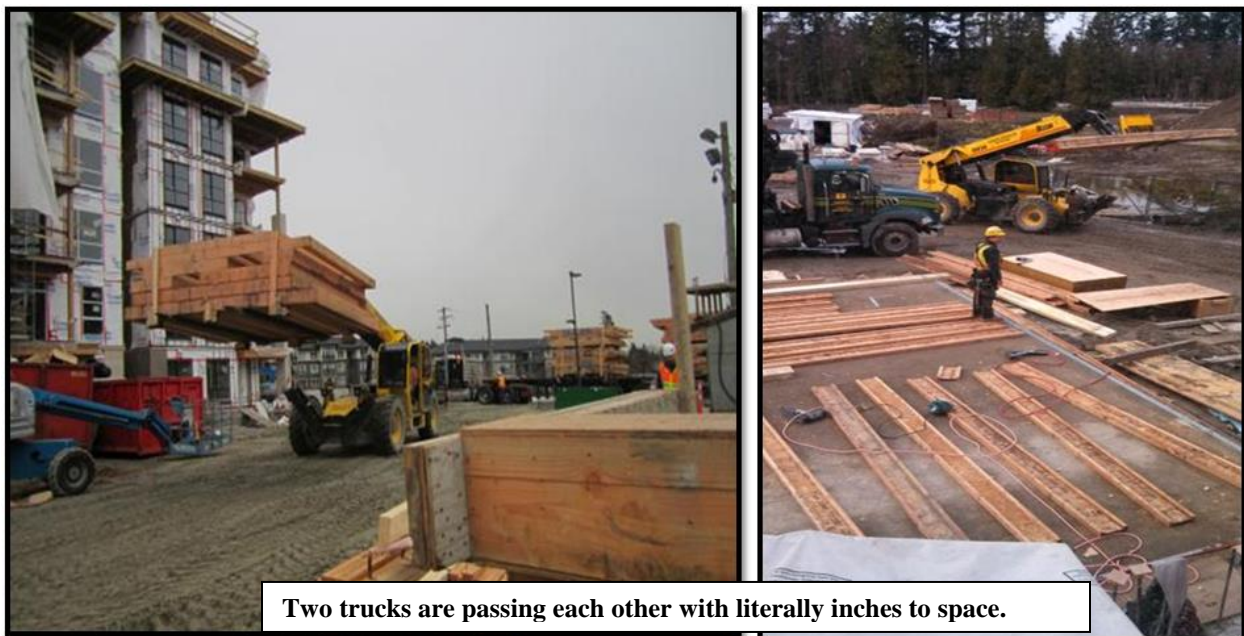
Figure 8: Safety Issue - Maneuvering of Large Equipment
