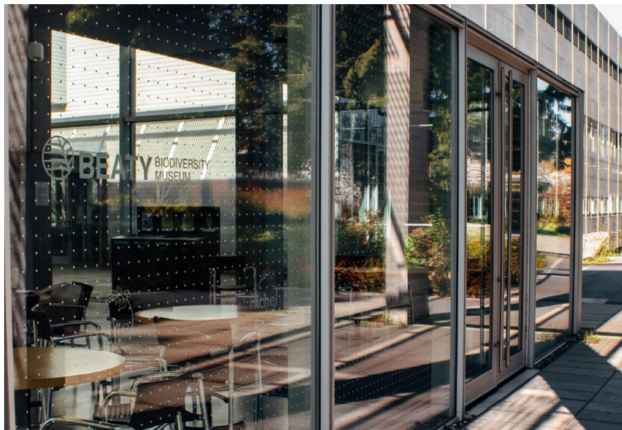
Figure 2. An example of FeatherFriendly® markers having been retrofitted on the facade of the Beaty Biodiversity Museum, located on the Vancouver campus of the University of British Columbia (University of British Columbia, 2019).
