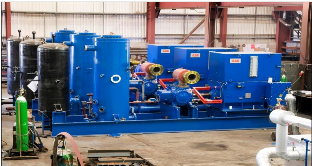
Figure 10: Star Refrigeration Heat Pumps in Drammen
