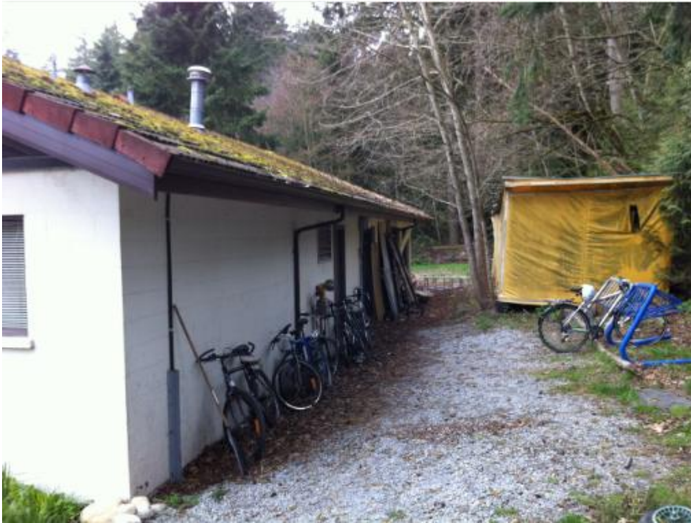
Figure 5.5 – Farm Center at the UBC Farm. A view of the gutters and drainpipes
