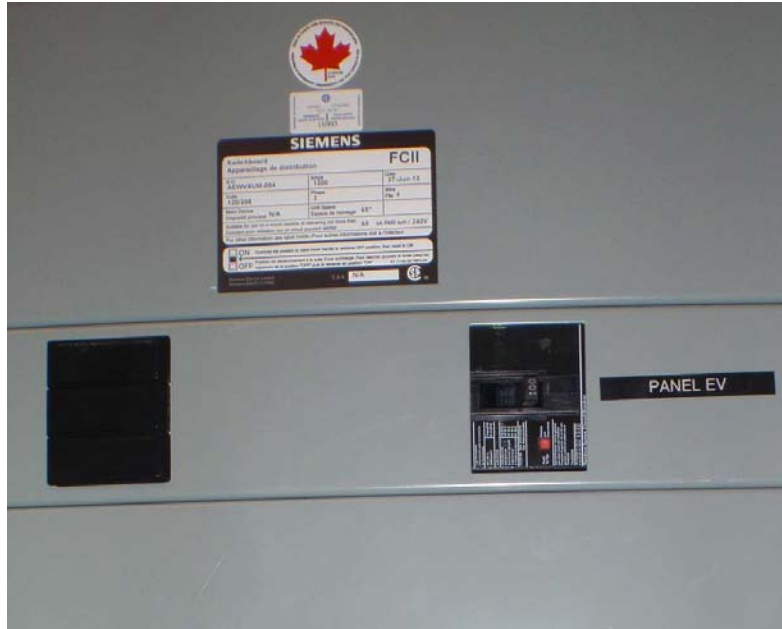
Figure 3 - Panel EV 100A Circuit Breaker in Main House Distribution Equipment
