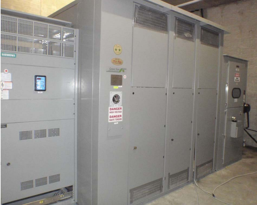
Figure 5 - Main Electrical Room - Incoming Switch and 1000 KVA Transformer
