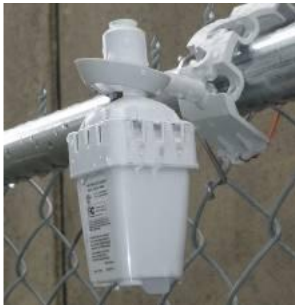
Figure 2: Water sensor currently in use at UBC
