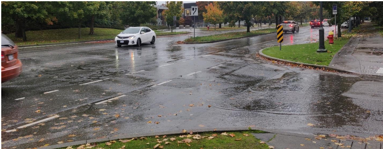
Figure 19 – Pooling at Existing RCMP Driveway Access
