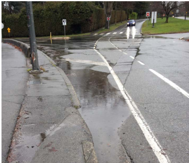
Figure 8: Water Ponding on SW Marine Drive - Photo Taken Jan 29
