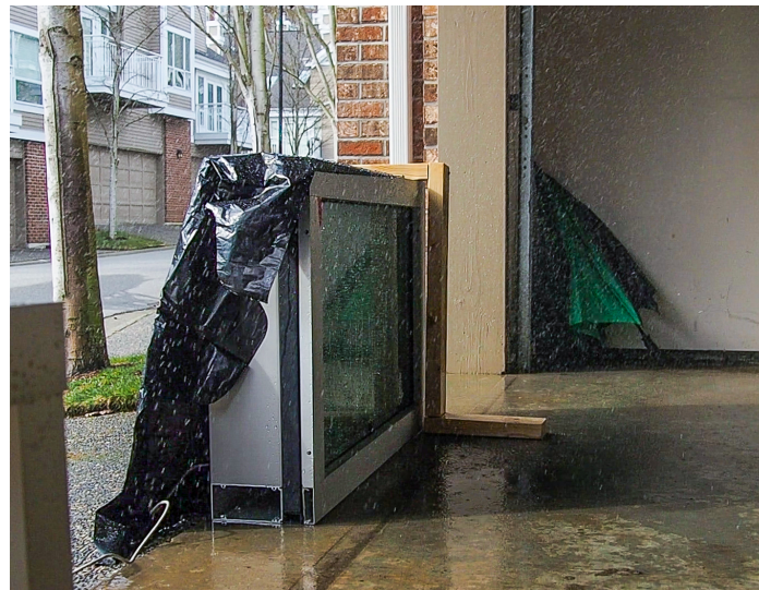
Figure E4: Window with Garbage Bag Sealing and Rain
