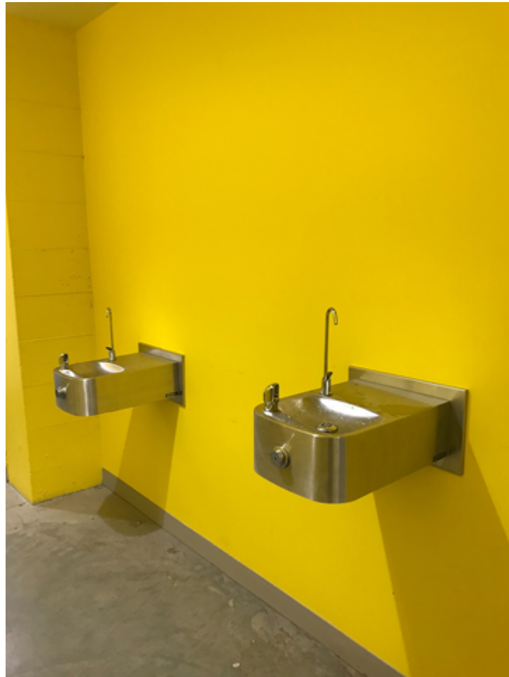
Figure 5 – LIFE building, floor 1, water fountains located in the washrooms behind the elevator (past Starbucks) – photo taken in the washrooms
