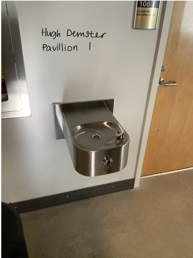
Figure 14.1 - Hugh Dempster, 1st floor fountain, photo taken facing towards the elevator
