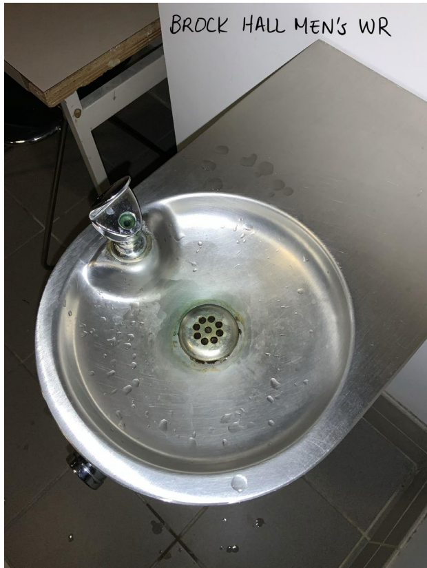
Figure 16.1 - Brock Hall, 1st floor by the men's washroom
