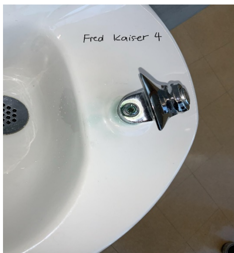
Figure 12.3 - Fred Kaiser, 4th floor fountain, taken at a different angle shows signs of oxidation on the bowl and the drinking spout.
