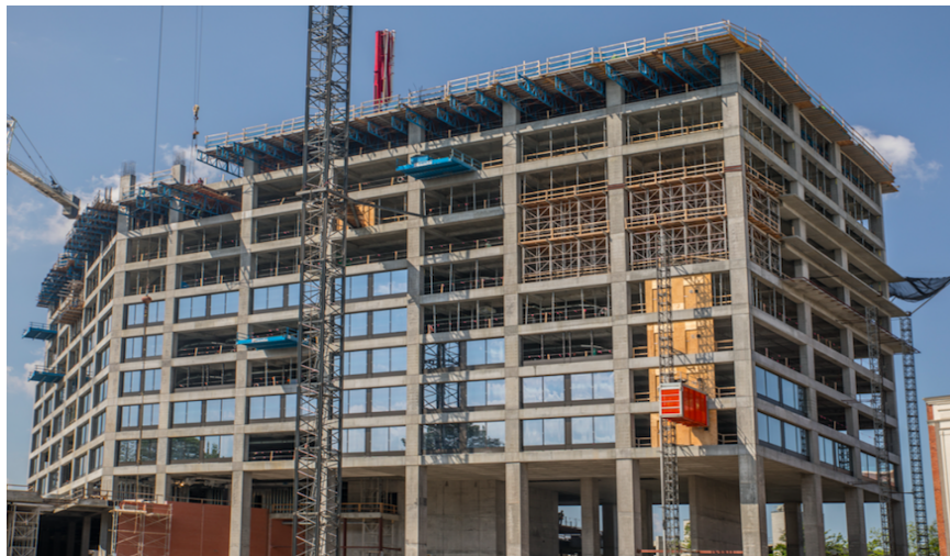
Figure 6 - 725 Ponce de Leon Ave in Atlanta. 365,000ft 2 – the structure built entirely with CarbonCure concrete [14]
