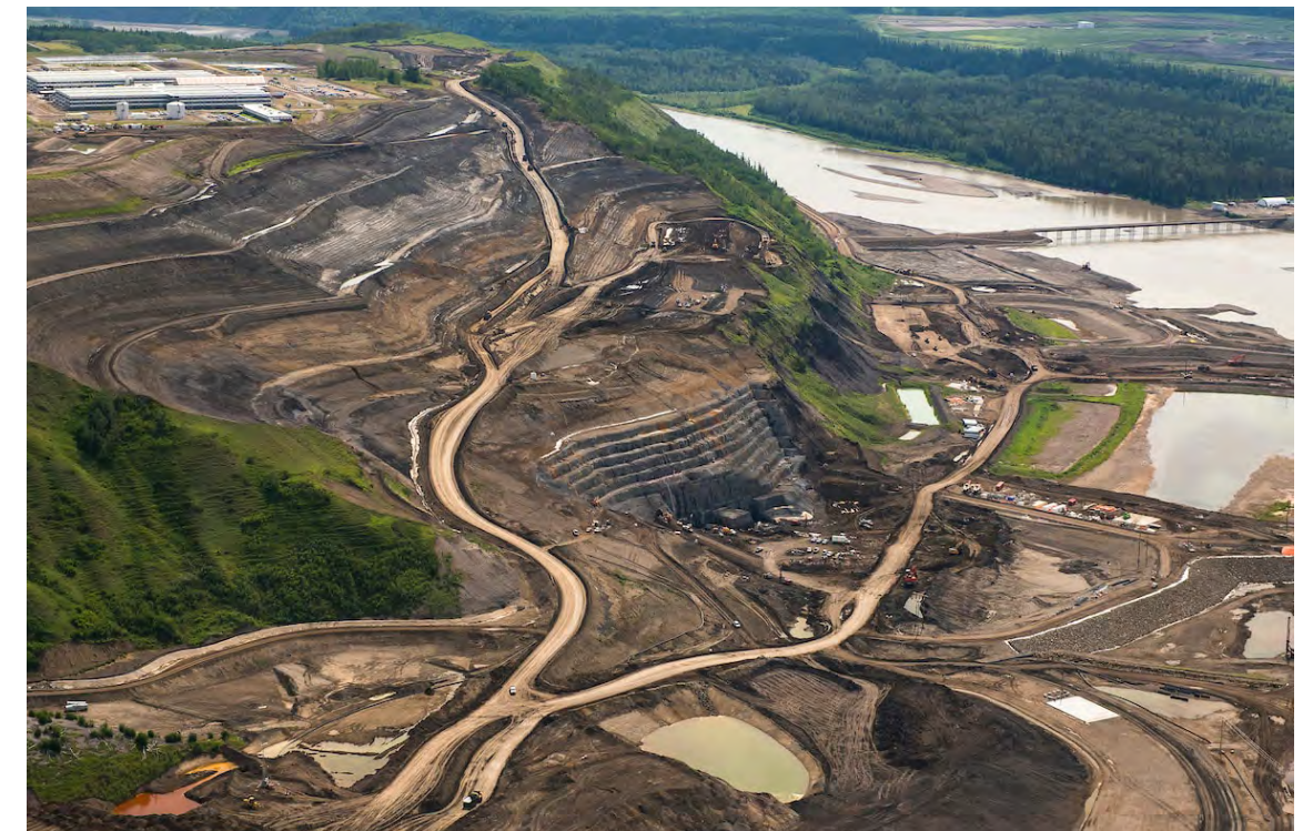
Figure 4. Site C Dam construction on the Peace River. © Garth Lenz for The Narwhal ( https://thenarwhal.ca/wp-content/uploads/2018/10/C2%A9Garth-Lenz-5443.jpg )
