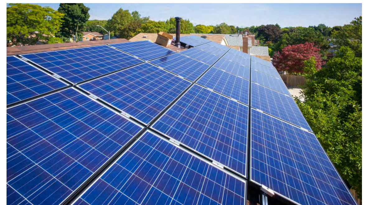
Figure 5. Solar panels mounted on building roof. © William F. Hertha ( https://hertha.ca/blog/2015924installing-the-solar-panels ). CC BY-NC-ND 4.0
