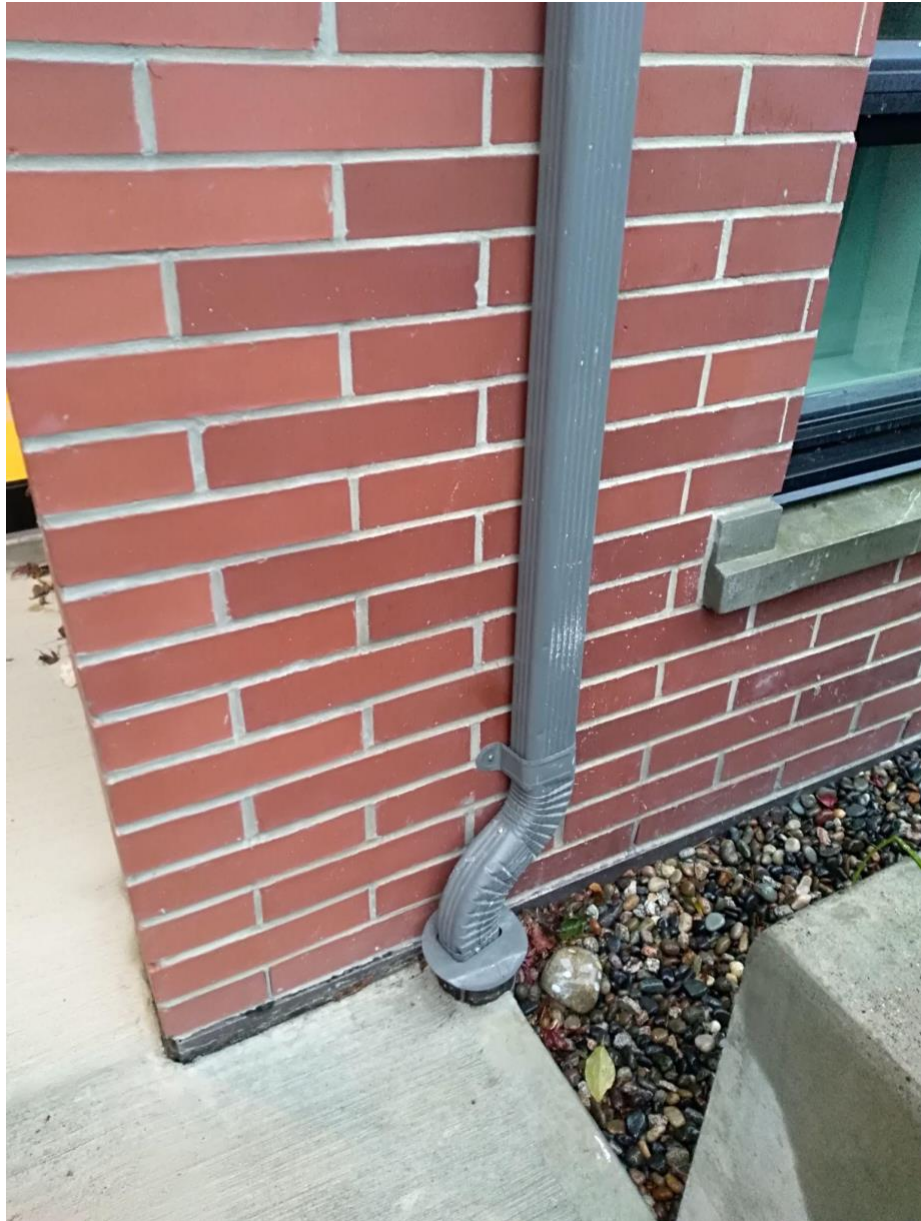
Figure 1. Drain Pipes at Webber House residence. [Photograph]. Larissa Santos.
