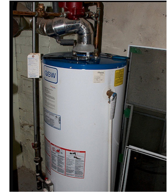
A residential hot water tank. Source: I am I.A.M.
