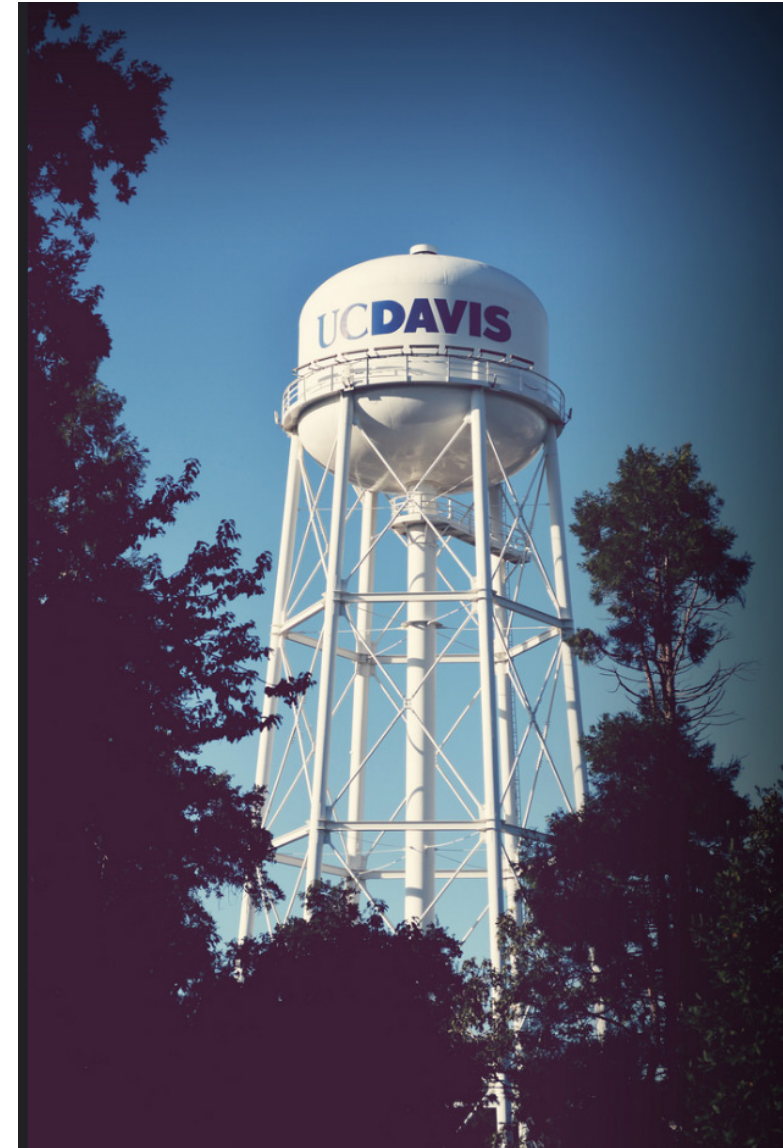
Bulk storage in a water tower Source: Steven Tyler PJS
