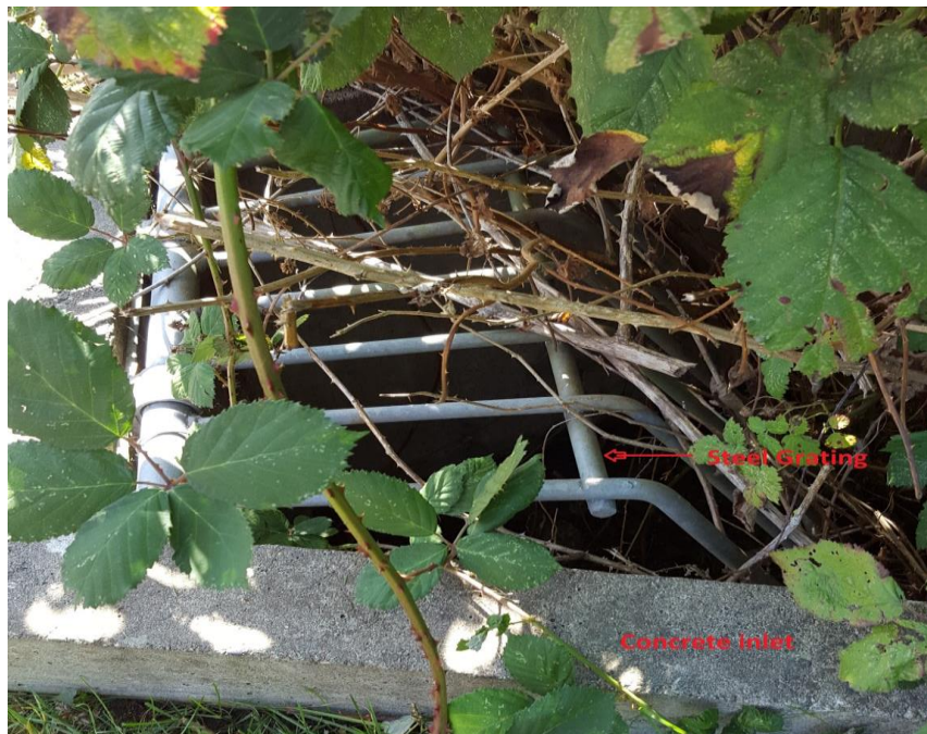
Figure 23 - Culvert Inlet at Wesbrook Mall, 200m North of SW Marine Dr. Intersection
