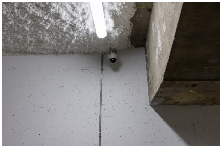
CCTV installed in all bicycle storage rooms
