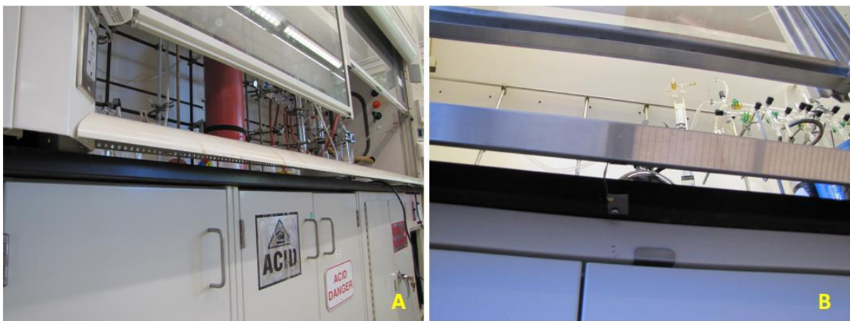
Figure 10 View showing the underside of VAV fume hood airfoils in (A) CHEM E and (B) CHEM D. This gap essentially maintains a minimum air flow in the event that the sash is completely flush (shut) with the airfoil.
