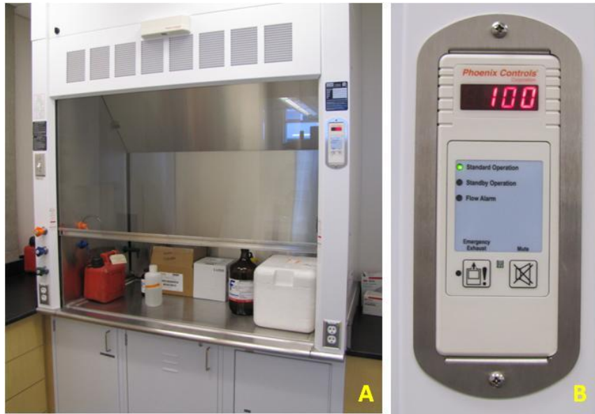
Figure 9 (A) Image of a state-of-the-art VAV fume hood in BIOS-W. Notable features include the motion sensor for room lighting (top), fume hood occupancy sensor (centre, above bypass grille), and controller (right, with red LED display). (B) Close-up view of controller showing 100fpm face velocity at standard operation (occupied condition). Standby operation typically reduces the face velocity to 60-80fpm (varies) when the fume hood is unoccupied. Flow alarm sounds when sash is raised above safe level such that complete containment is not guaranteed.
