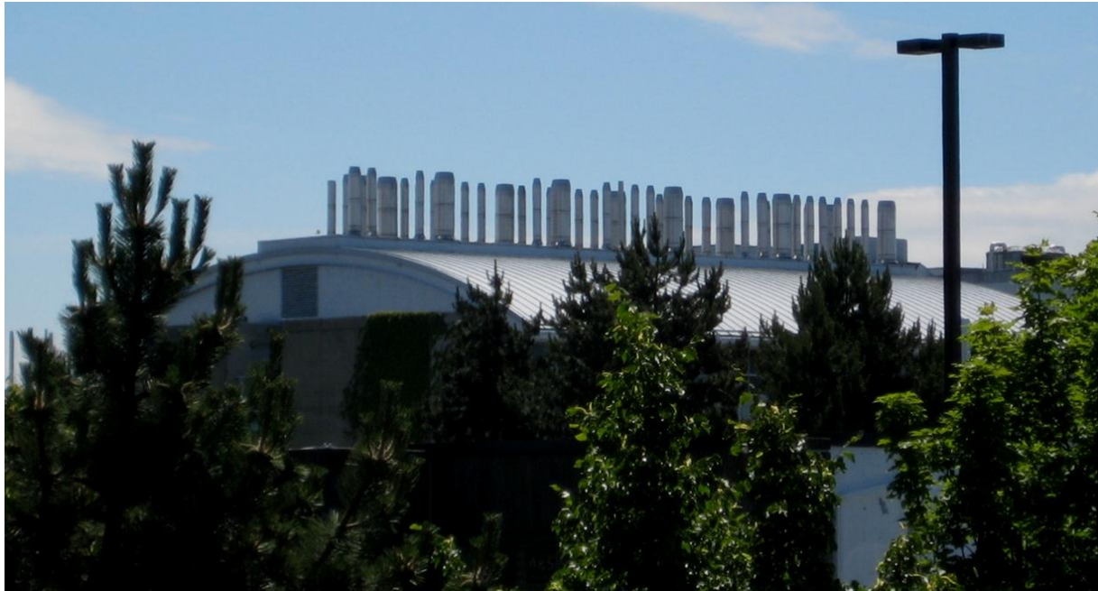
Figure 4 Exterior / roof level of the AMPEL building. Each fume hood has a dedicated stack with an additional 13 general exhaust stacks (~50 stacks total).
