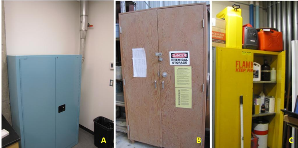
Figure 7 Chemical storage cabinets like these are regularly found in laboratories; however, during the audit only (A) BIOS-S had dedicated ventilation ducts that connect to the HVAC system directly – (B) and (C) represent all other cabinets observed that vented naturally to the ambient laboratory room air.
